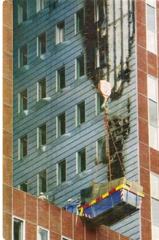
Details are important! Unless warnings from the roofing constructor they choose the cheaper detail. Result; the wooden substructure caught fire.
